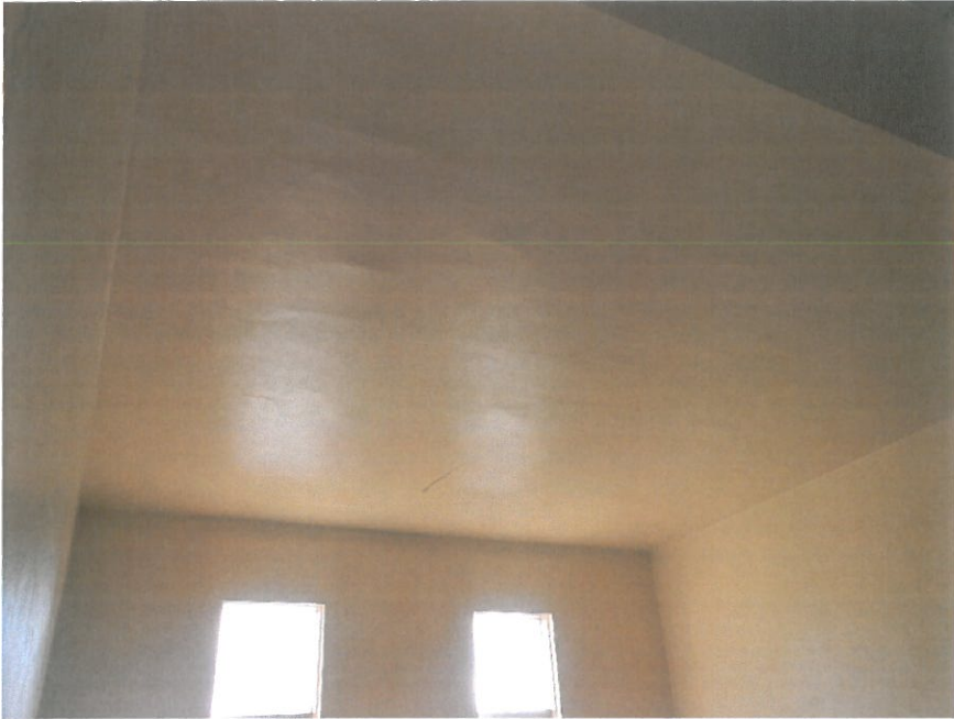
This photograph illustrates another section of the ceiling and its cracking.
